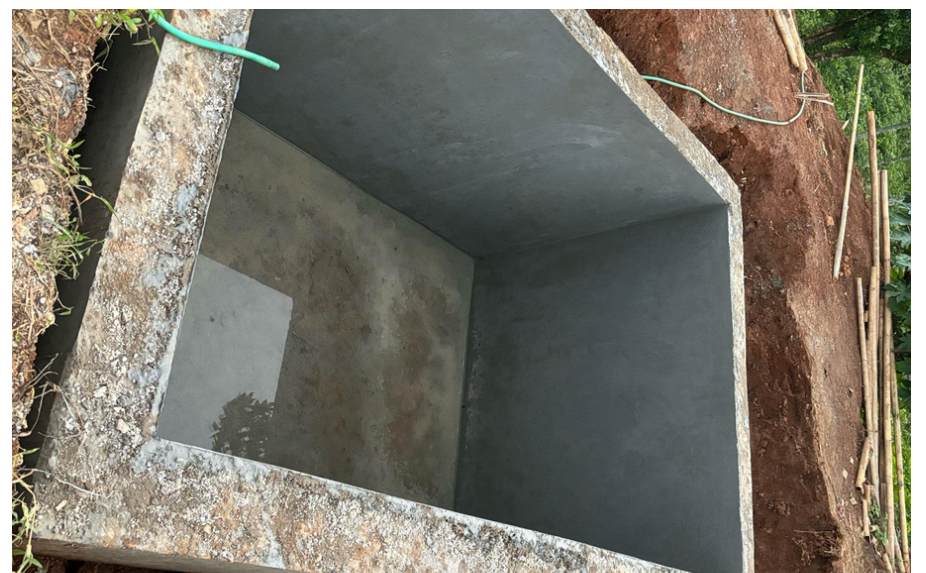
Progress of Rainwater Harvesting Tank in Asil Songgital village Under Songsak Block.
